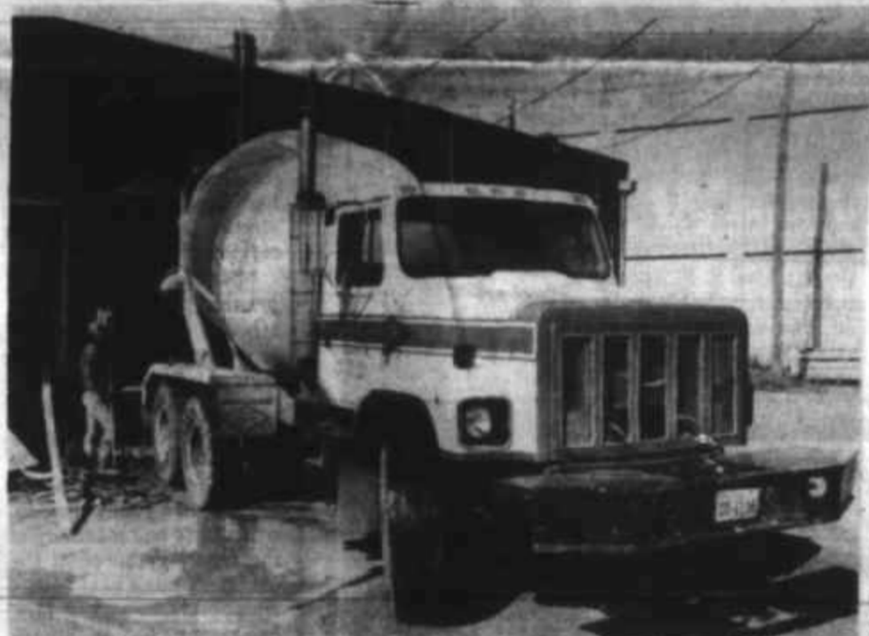
Cement trucks brought in a new floor for the space next to The Headlight where Connie Herman is opening a new restaurant. The name will be Lone Star Pizza and Sandwich Shop, and the opening is planned in about five weeks.
